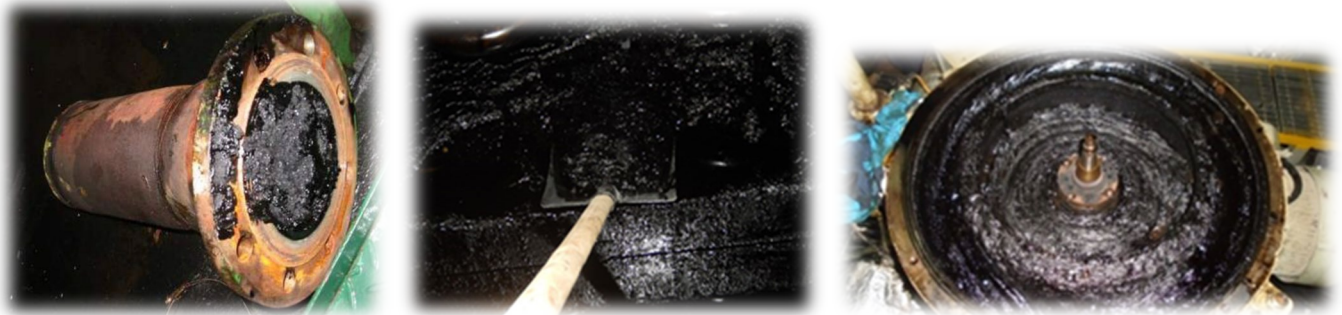
Figure 1: Examples of asphaltenic sludge precipitation
